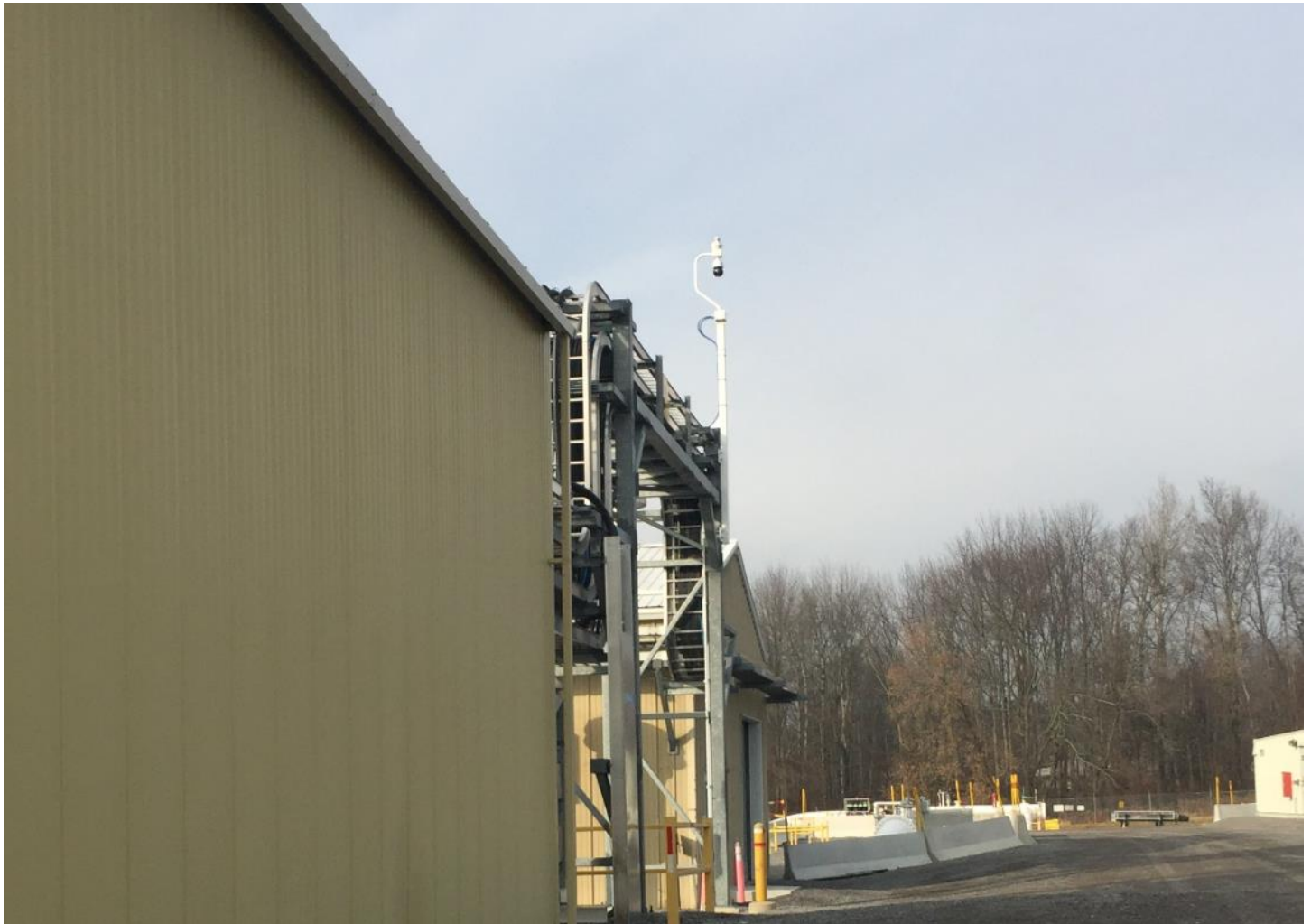
Object 1: Mounted Thermal Radar Hydra using an Axis Q6155-E PTZ on a 15 ft pole.
